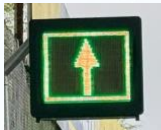
Track side panels
